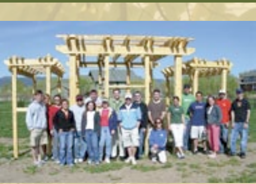
Left and above: Students build shade structures for community gardens using wood thinned from Colorado forests.
